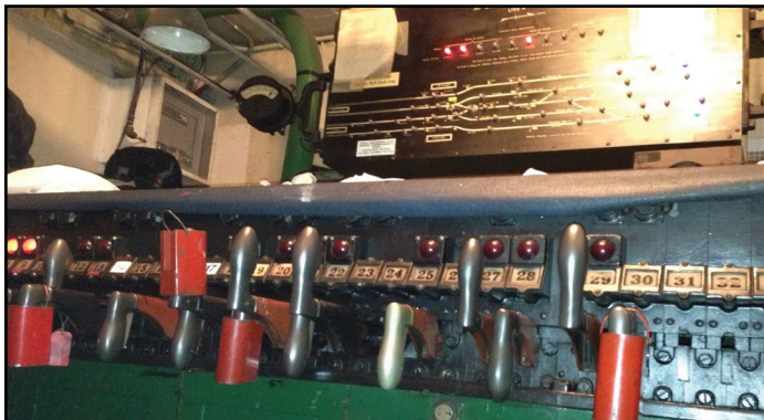
Lever style electro-mechanical interlocking machine at 30 th St. on the Eighth Avenue Line. Similar to the US&S Model 14 board, here the top levers move the switches and the bottom levers control signals. The red cans over a lever are lock-outs.
