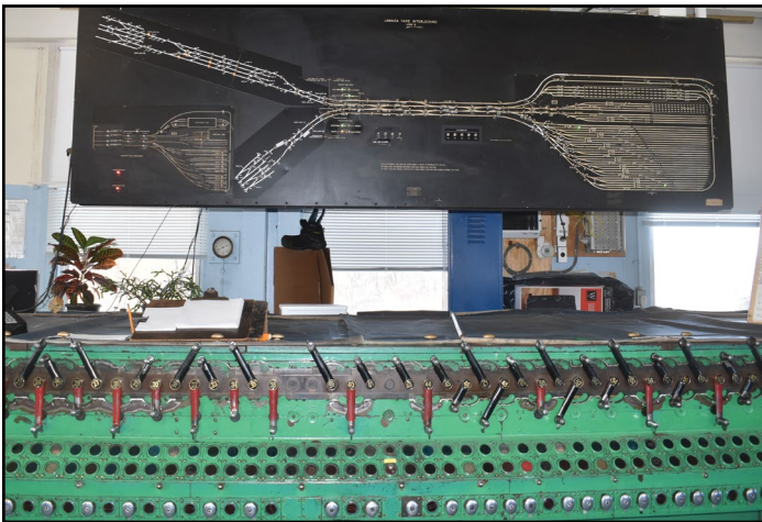
Jamaica Yard interlocking machine. Switches are controlled by the upper levers (normal to the left, reversed to the right), and signals by the lower controls. Red signal levers can be swung left or right of center, which would correspond to signals X-L60 or X-R60 being permissive in the case of lever 60. Facing straight down, both signals would be red. Black signal levers are either permissive (right) or normal (red). Here switches 23, 29 & 31 are reversed, all signals are at danger (red).
