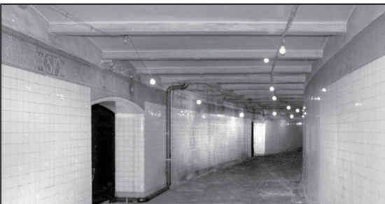
Abandoned Inner loop station platform, although longer than the outer loop, is too heavily curved for regular operation. In fact, when the last passenger trains serviced the Inner Loop in 1977, only the center doors of the cars in shuttle service could be opened and they mated with alcoves cut into the walls.
